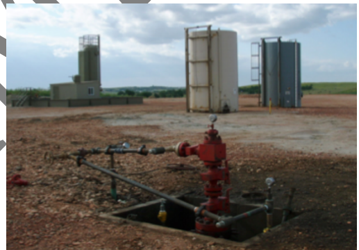
Wellhead left after fracking equipment has been removed. Photo credit: Joshua Doubek
