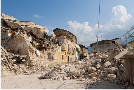
Earthquakes can damage buildings.
