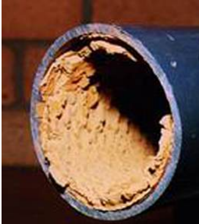
Mineral buildup inside a water pipe
