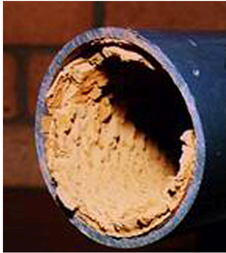
Mineral buildup inside a water pipe
